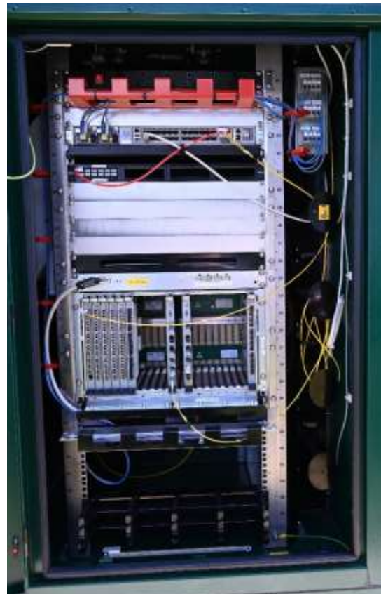
Figure 1: Typical new-build cabinet, populated with Gigaclear equipment - for third-party use this rack is empty from U21 down
